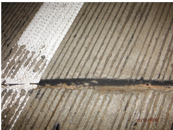
Photo 5. Black Expansion Joint Material
